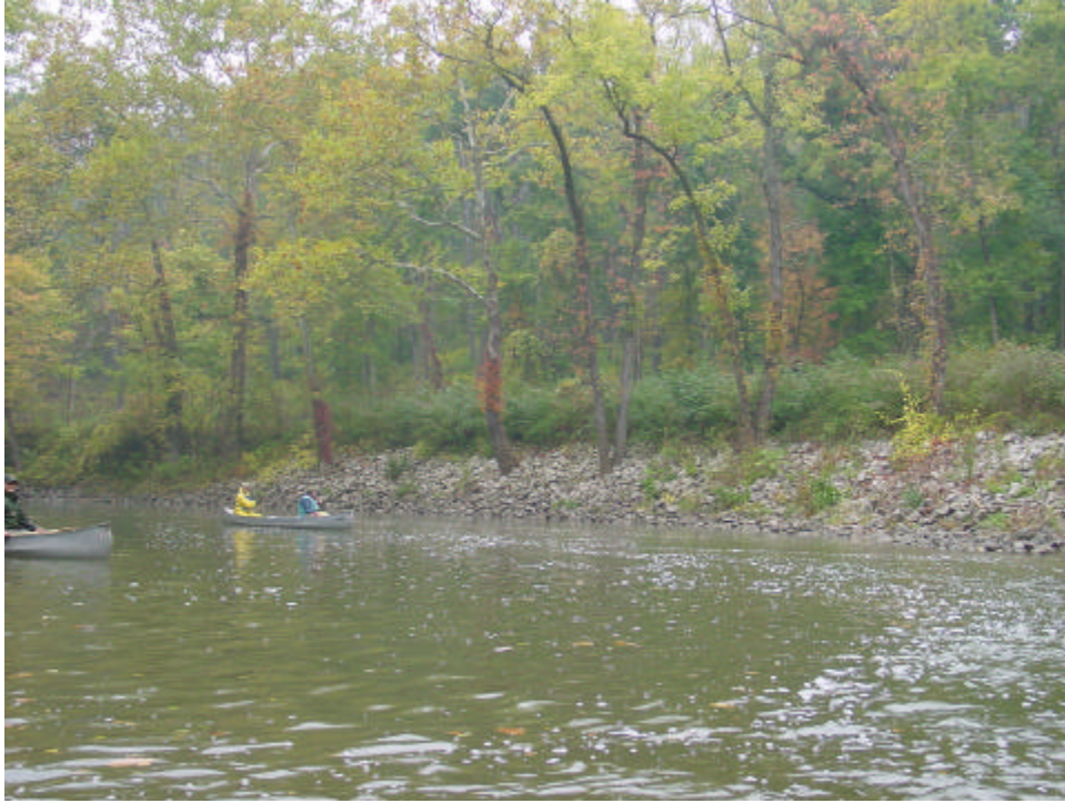
Figure 9. Careful placement of riprap can allow the preservation of mature trees along the banks and avoid impacts associated with their removal
