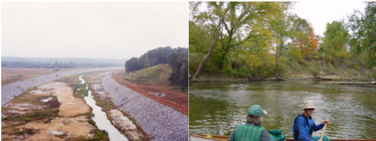
Figure 3. Common problems include setting the riprap elevation higher than needed and not extending the protection far enough downstream
