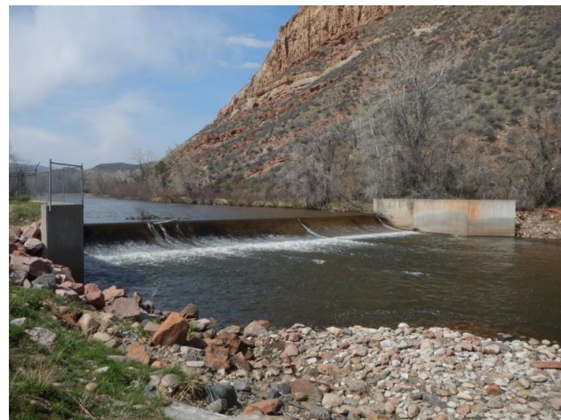
Figure 4. Diversion structure at the Watson State Wildlife Area, Cache la Poudre River.
