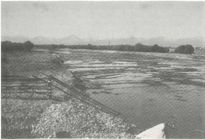
CHANNEL CLEARING AND DIKING ON BIG HOLE RIVER. Nearly one-third of this excellent stream had man-made channel changes.
