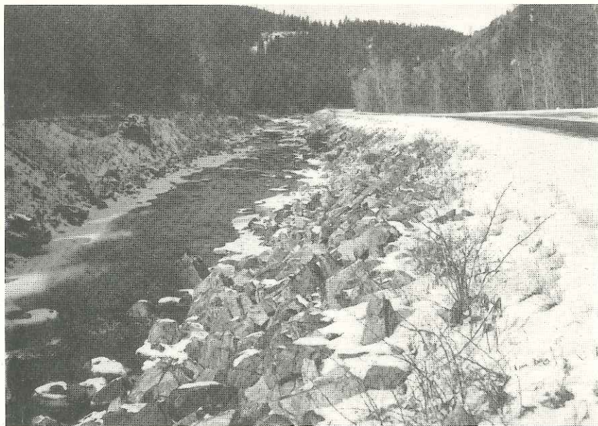
A STRETCH OF RELOCATED CHANNEL RIPAPPED INTO PLACE. Belt Creek near Great Falls had 26% of channel altered.
