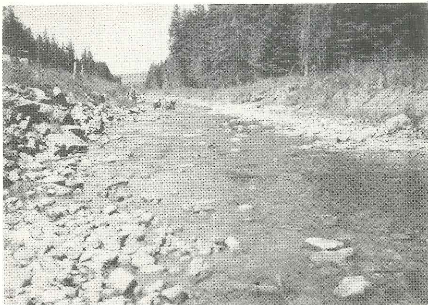
A CHANNEL RELOCATION ON SHEEP CREEK NEAR WHITE SULPHUR SPRINGS WITH RIPRAP USED TO MAINTAIN THE STREAM-BANK. Nearly one-third of this stream had been altered.
